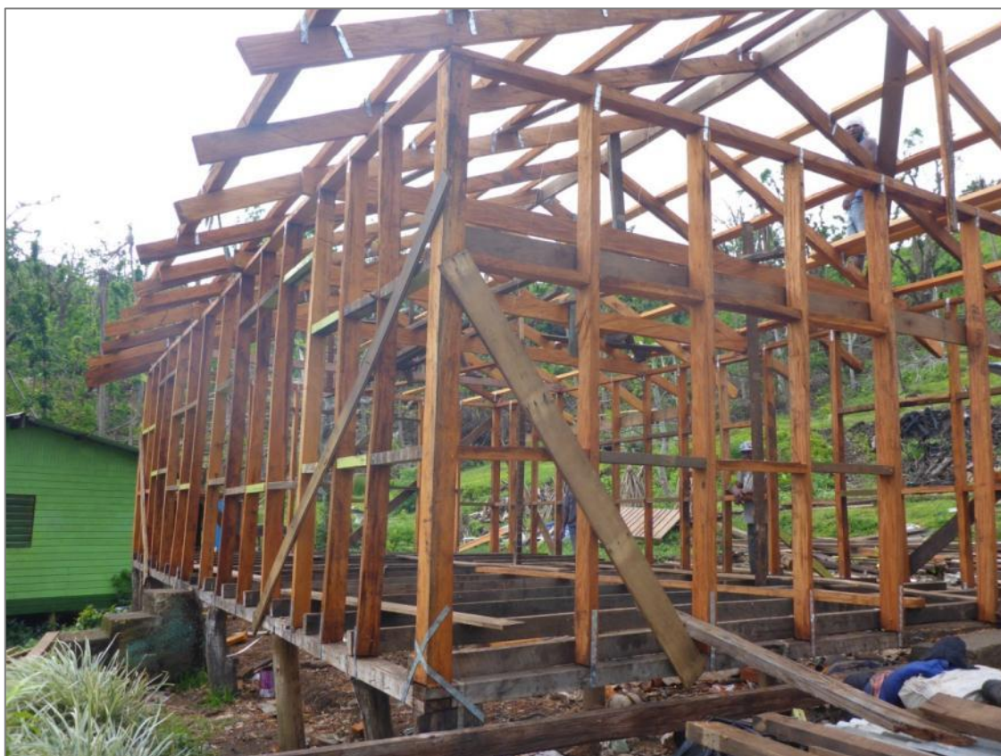
Figure 6 – House being constructed with locally processed mahogany timber – Verevere (photo credit: Camille Laude)
